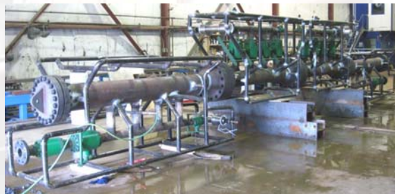
White Rose North Amethyst Subsea Production Flowlines Pig Launchers and Receivers
